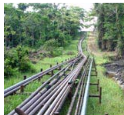
Achuar territory in River Corrientes is criss-crossed by a web of aging oil pipelines, many of which slowly leak crude into the surrounding jungle.
