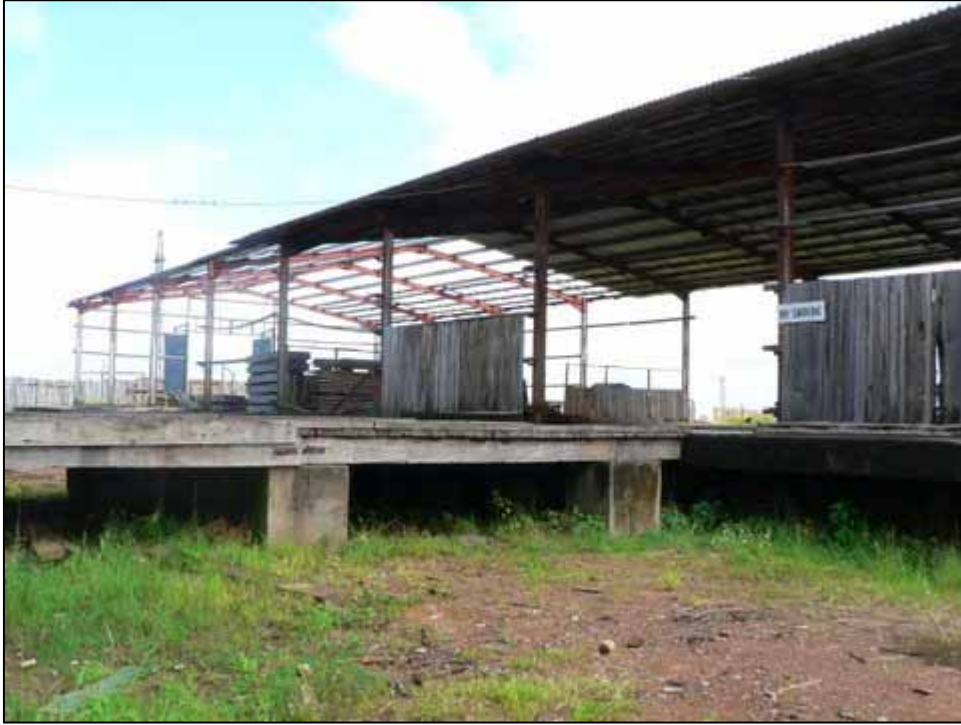
The former OTC sawmill at Buchanan harbour. Now under the ownership of a Spanish company.
