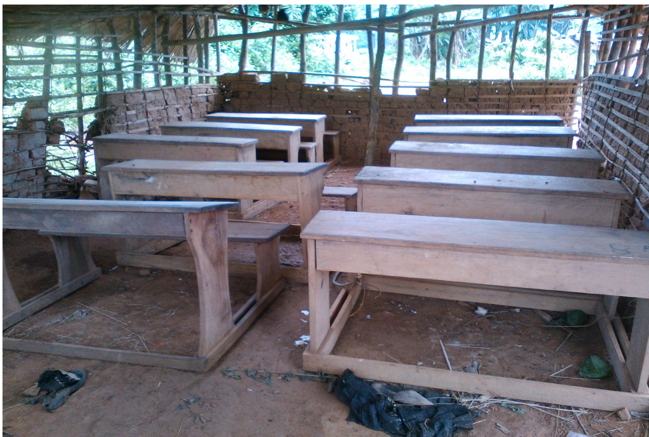
Dilapidated school in Assoumindélé II which ought to be able to house a hundred children
